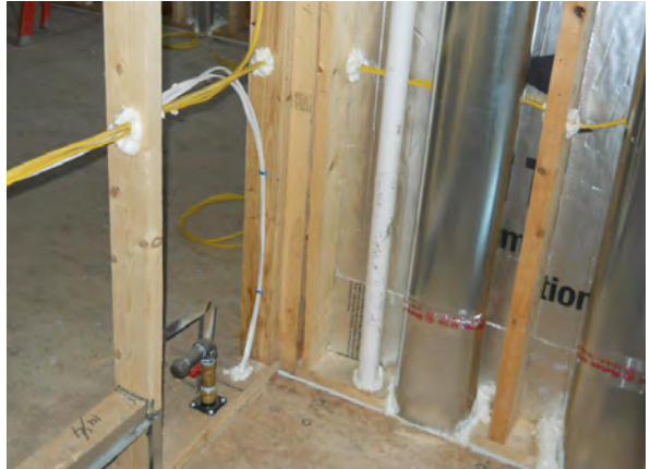
Plumbing, electrical and HVAC penetrations between floors.
