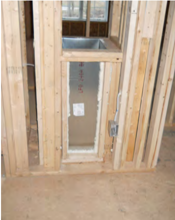
Duct chase between floors.
